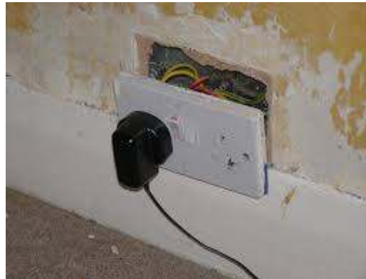
Improper loose connection
