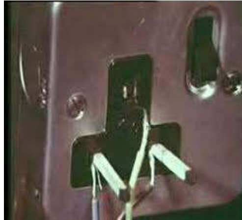
Loose wire connection using match stick
