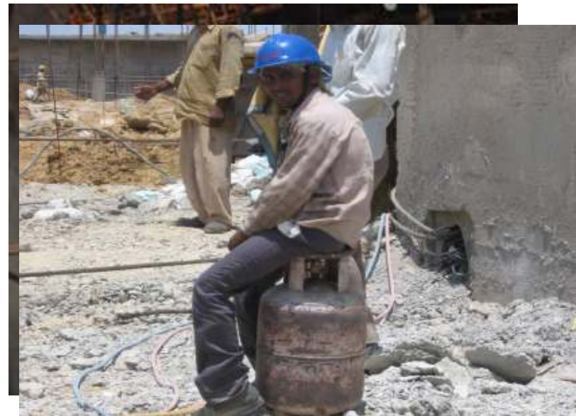
Bad illumination Unsafe practices
